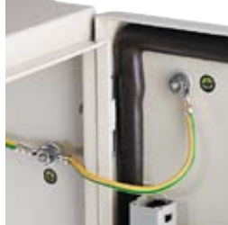
The earthing studs are welded to the door and in the body.
