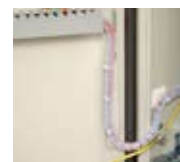
Cable management devices
